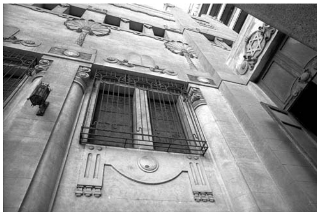
Figure 5. The "Gate of Heaven" Synagogue, Cairo. Facade, "Sun" discs and other decorative motifs, details.
